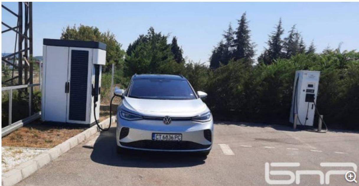
Figure 10 EV charging point at Audi showroom in Stara Zagora
