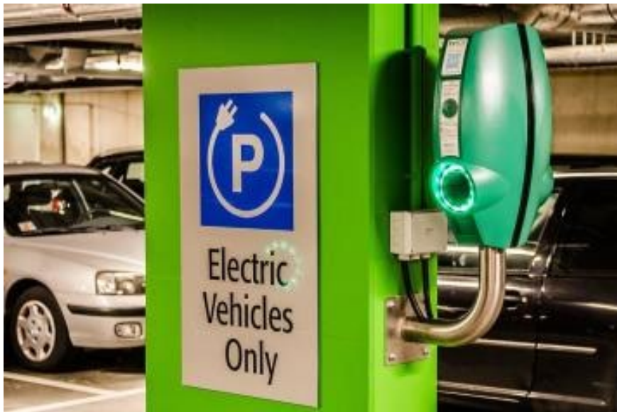
Figure 14 EV charging point to promote sustainable mobility
