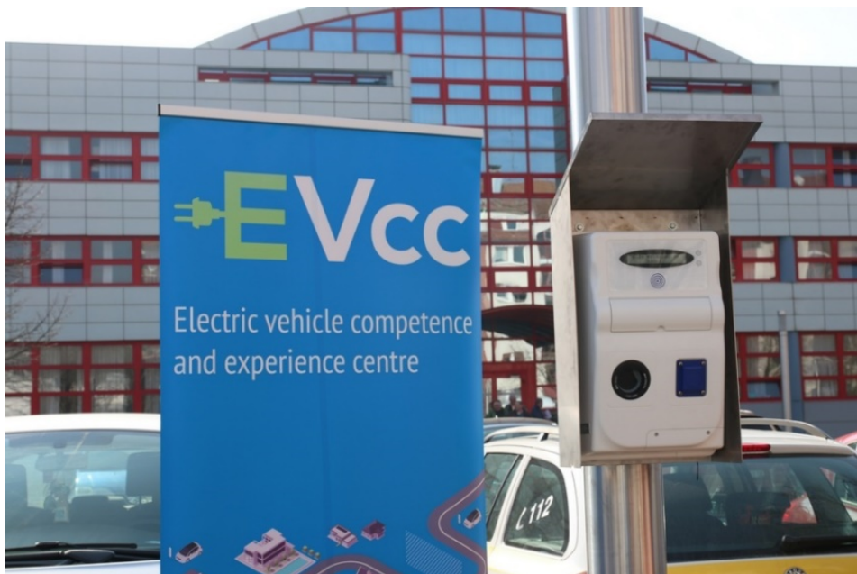
Figure 6 EV charging station on the lamppost
